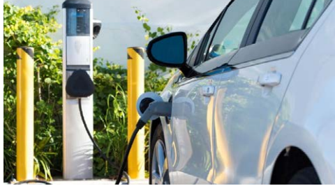
EV Charging Stations
